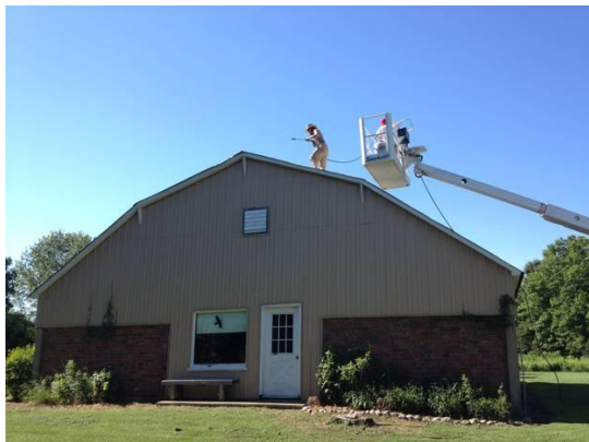
The Bremer Sanctuary barn roof gets a face-lift with some much needed repairs and a new paint job. Photo by Don Krefft.
